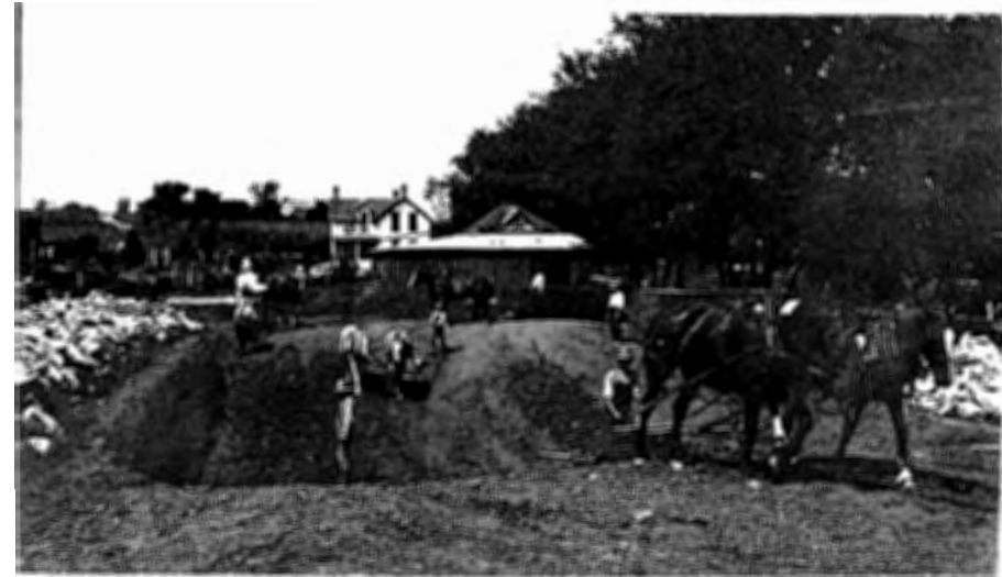
New store 01: Four teams of mules pulling slips excavate the basement for the new Kratzer Bros.' store at Volland in this Otto Kratzer view from the summer of 1912. (Courtesy Wabauunsee County Historical Society)
